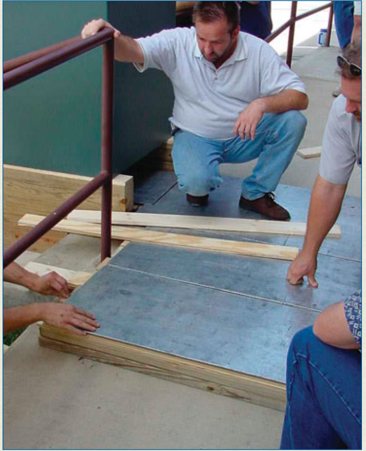
5. Leveling the platform on a downward incline so the safe can be moved up or down safely.
